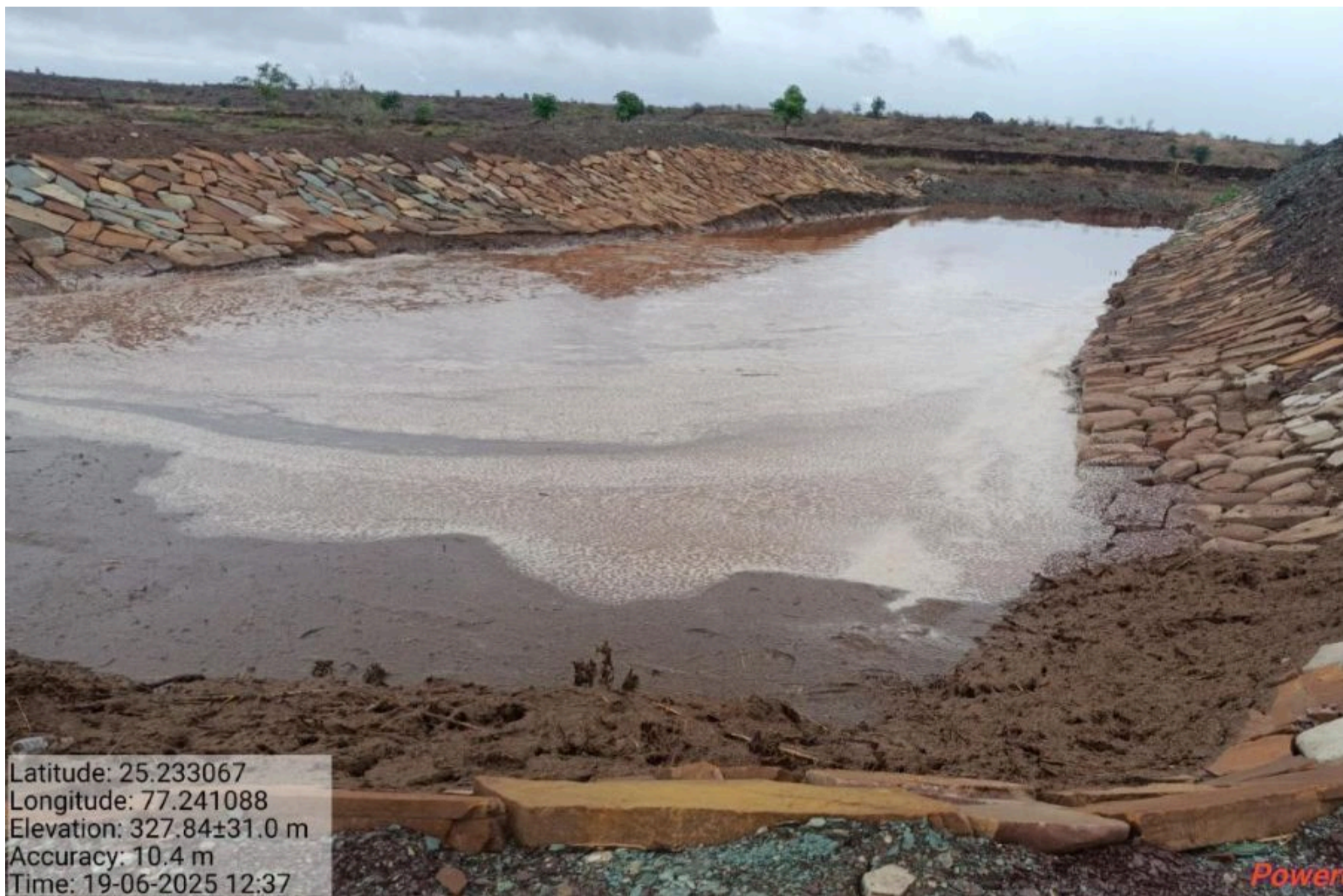
The newly constructed farm pond begins to collect water, paving the way for irrigation support and groundwater recharge
